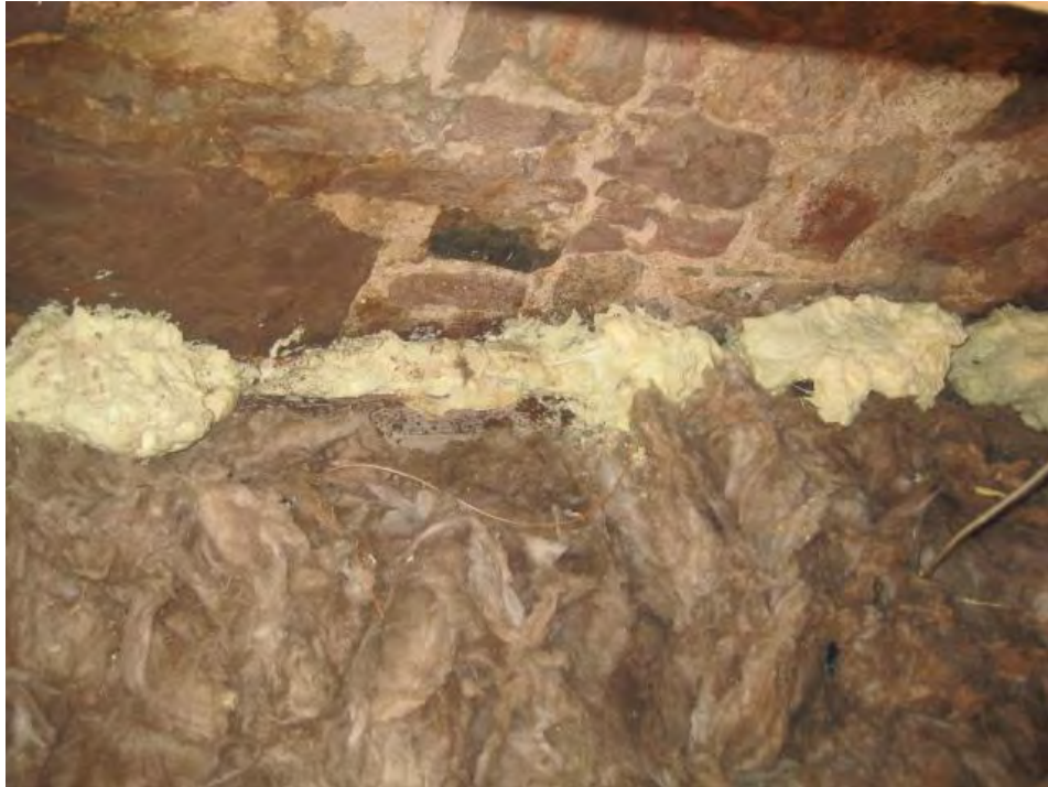
Top of the gable wall, foam seen from the attic
