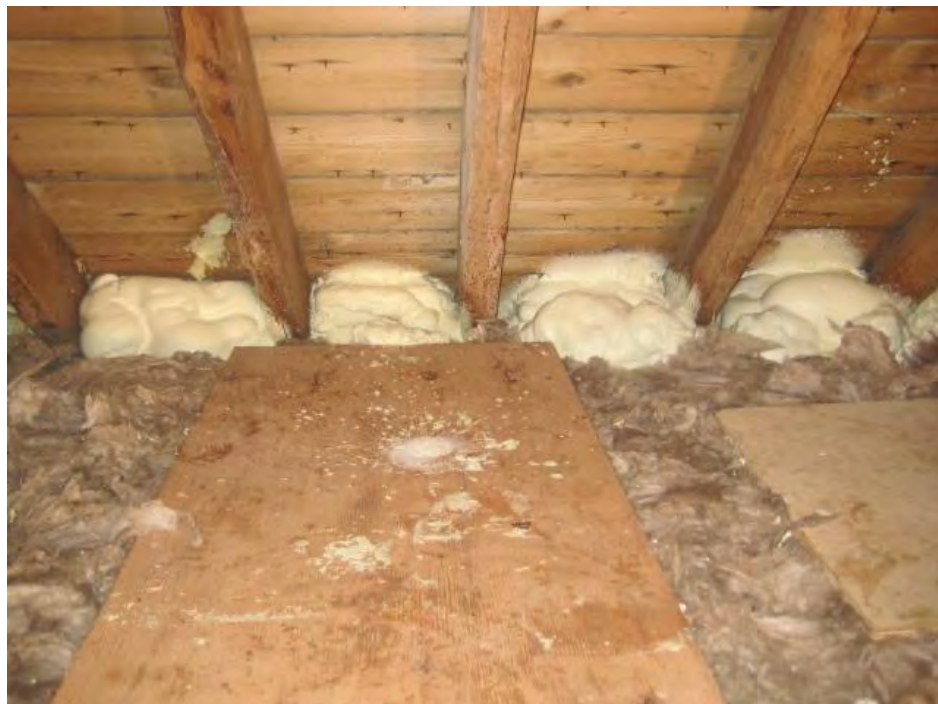
Foam seen at the eave level
