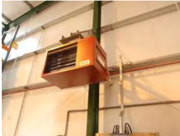
Fig. 03 Combat air heaters in the warehouse
