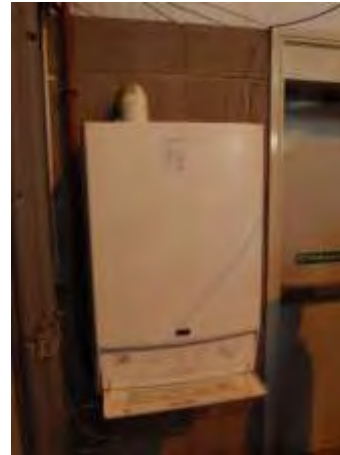
Fig. 04 Conventional Gas boiler
