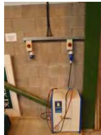
Fig. 07 Forklift charge up station
