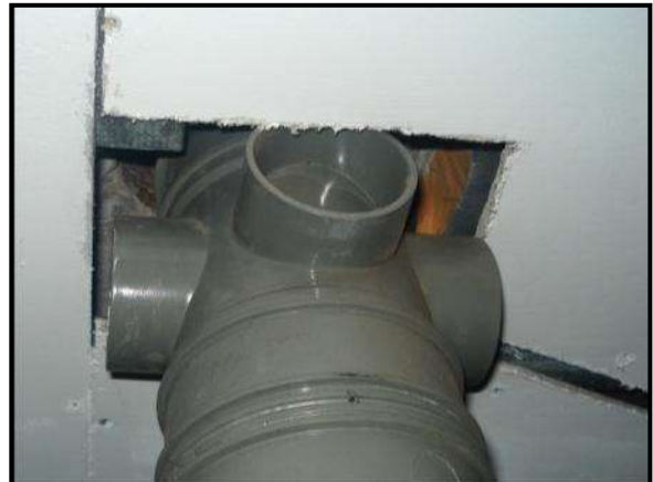
Figure 09 – Source: CJ Walsh – Consultant Architect, Fire Engineer & Technical Controller
