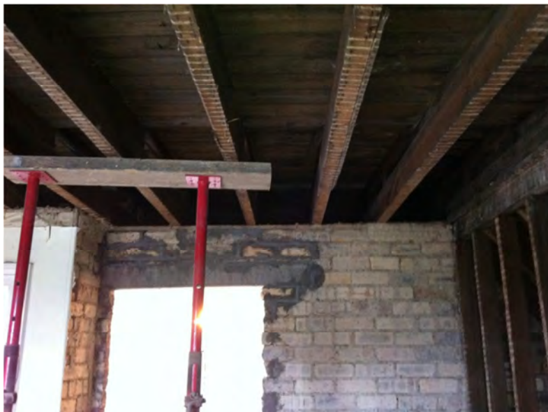
An attic space undergoing alterations, exposing the existing rafters. Grigor Mitchell Architect Ltd.
